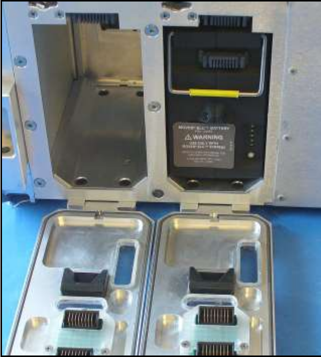
Figure 9-10: Battery Disconnected (compartment open)
